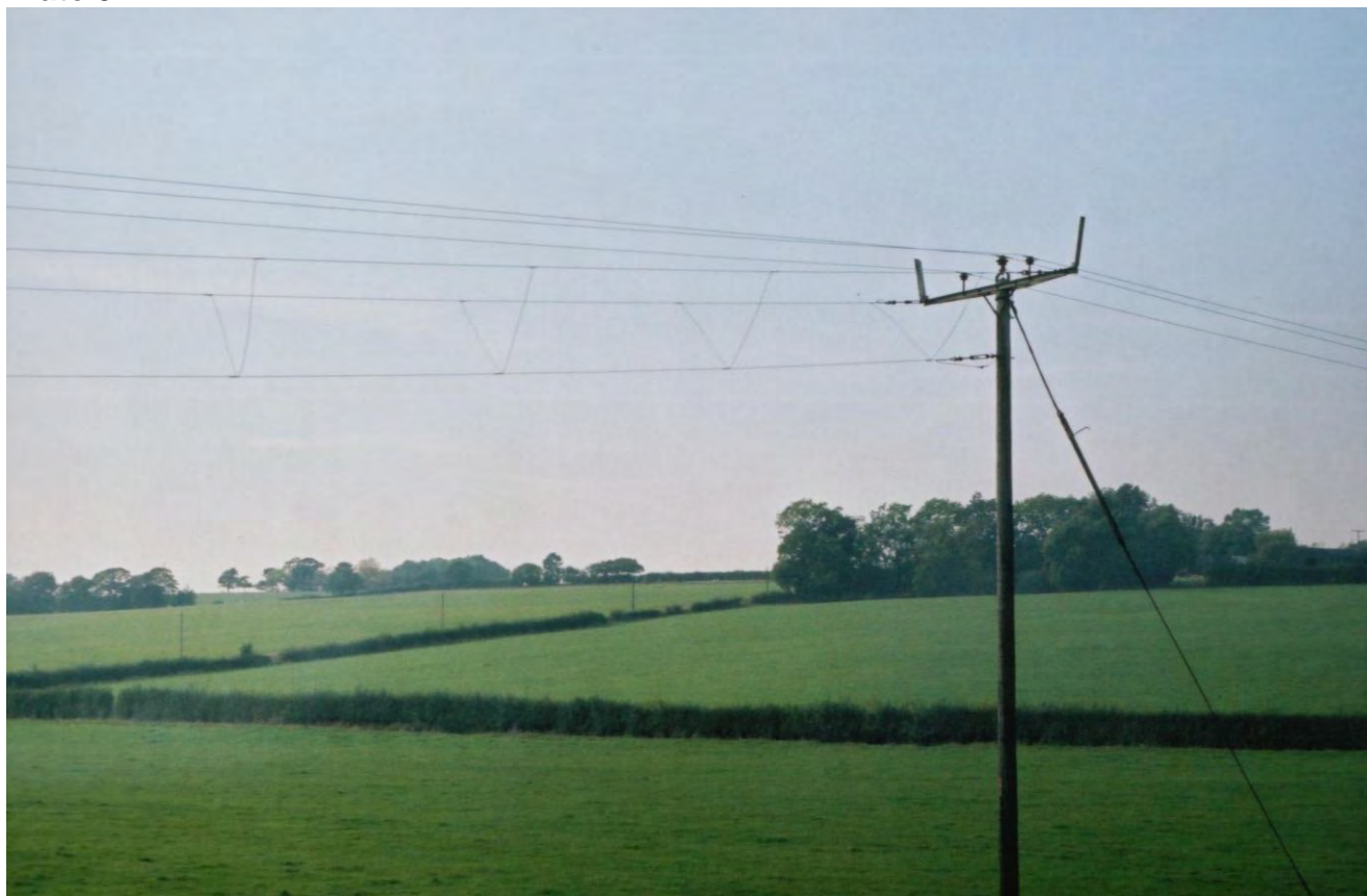
Shows a post 1959 cradle guard with insulated stays crossing the Kent and East Sussex Railway on 28 th September 2001. This is a South Eastern Electricity Board design.
